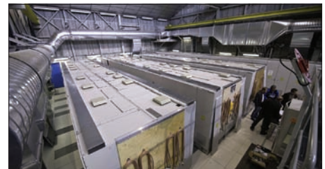
The new PS power-supply system is made up of six containers, each with 60 tonnes of capacitors and eight power converters.
